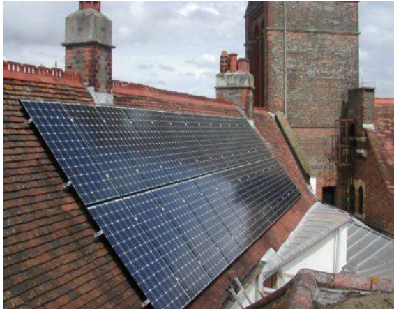
26 Solar Photovoltaic panels
